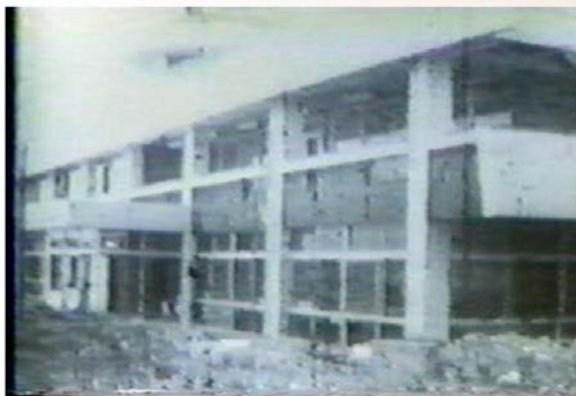
1964 Niigata Earthquake: Sinking terminal building
